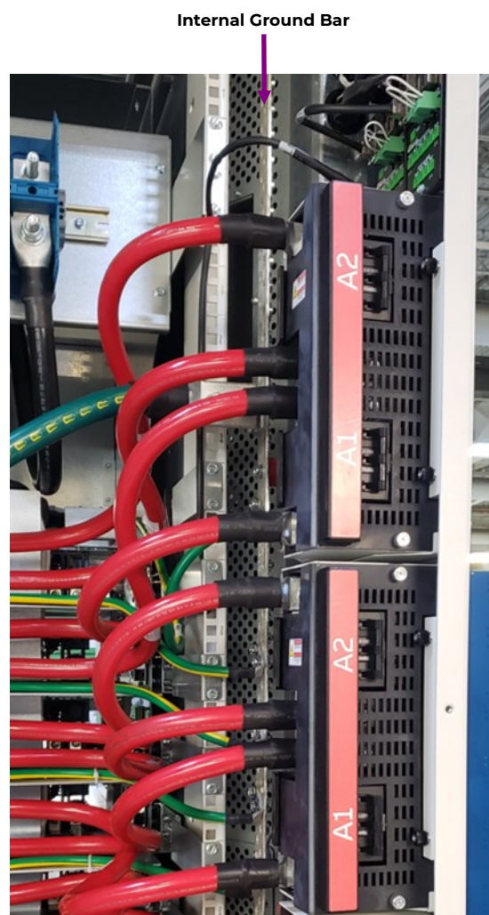
Figure 10 Internal Ground Bar
