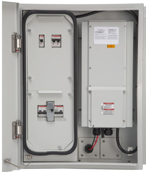
AC Input and CC1600 rectifier compartment
